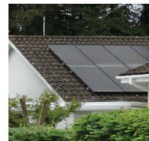
Roof solar panelling.
